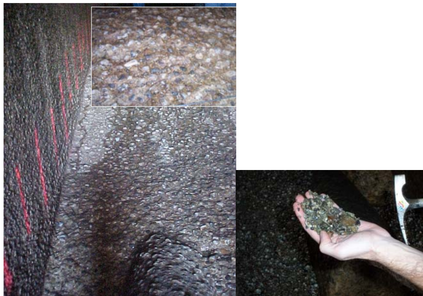
Figure 2. — Typical abrasion damage (Choke Canyon stilling basin).
